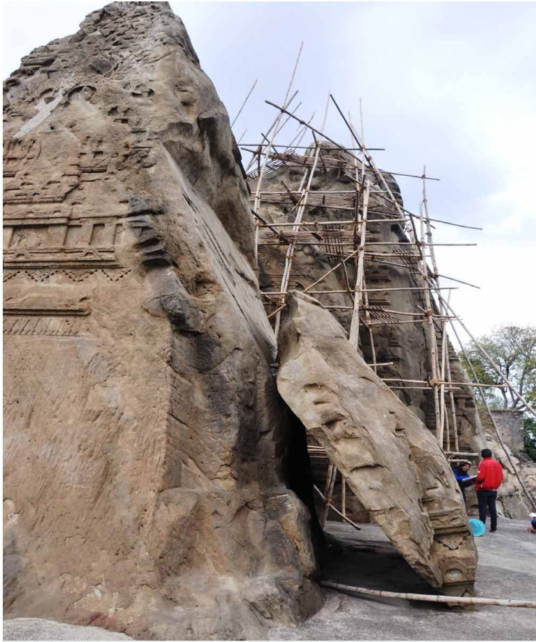
fig. 34 Fallen portion of shikhara
