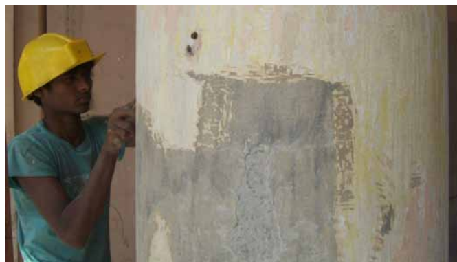
fig. 32. Cement based repairs that caused accelerated decay to the century old brick structure
