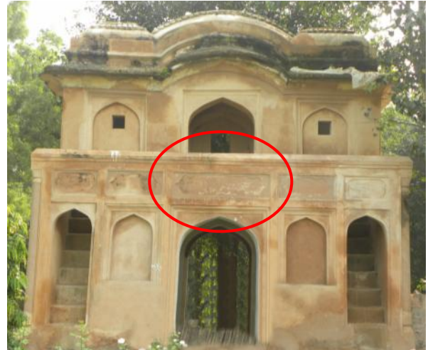
fig. 2 Gateway, Lodhi Garden: Dampness on the walls due to non-existence of water drainage system
