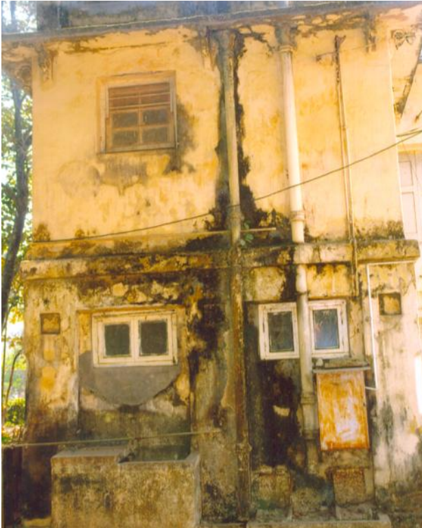
fig. 4 Effect of rainwater pipes failure in a modern structure
