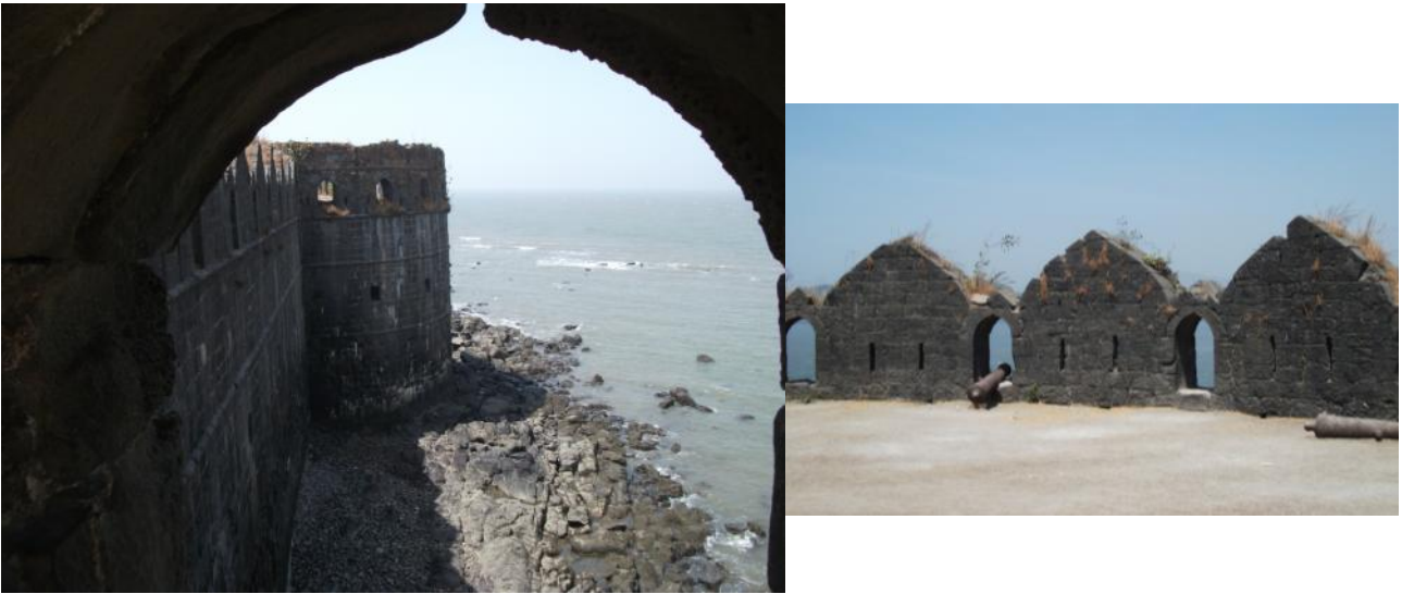
View of the outer wall (left); battlement wall now covered with vegetation (right) (source: Harish Benjwal, 2012)
